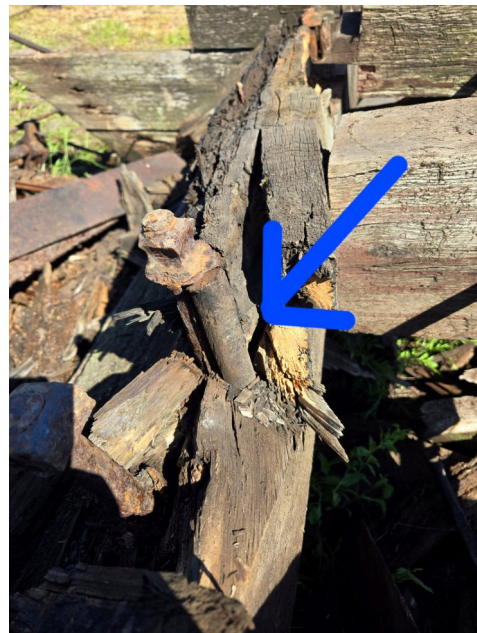
Portion of one of #36's frame cross beams, showing the dowel used to plug an incorrectly drilled hole. Note the bolt next to it, which is in the correct position. This was one of the eyebolts that acted as a hinge for the car's hopper door.
